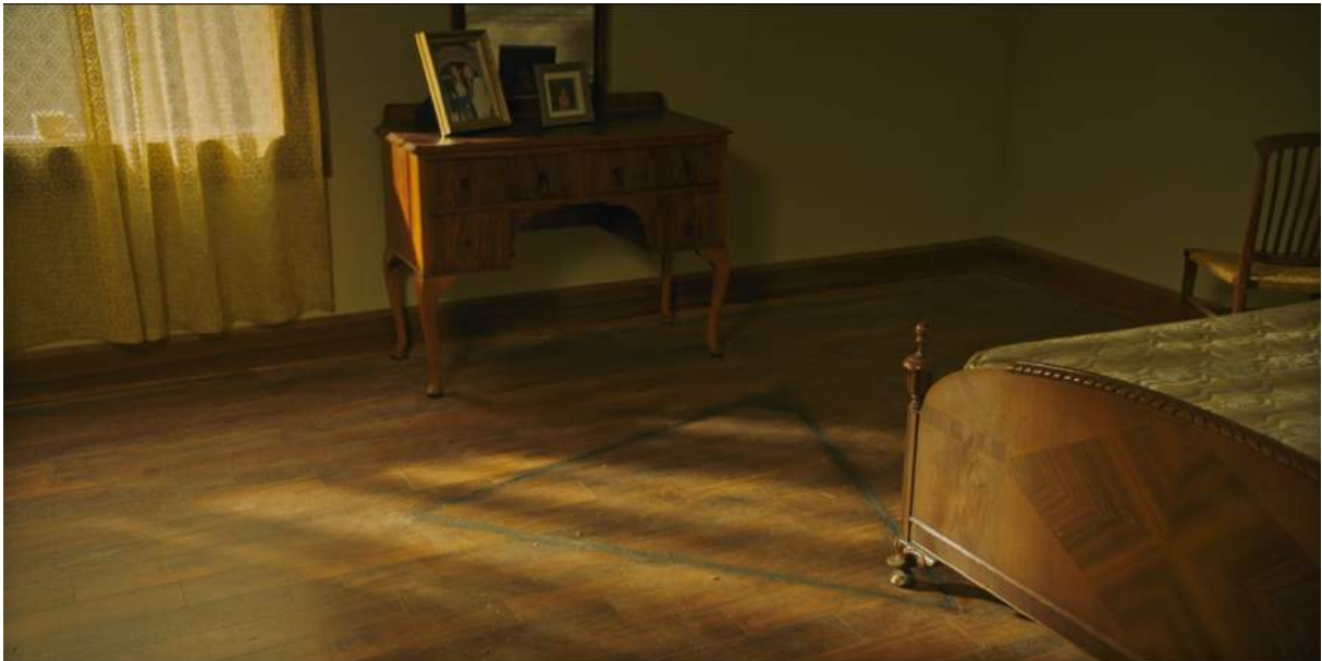
Figure 17 – View of the triangle burned on the floorboards.
